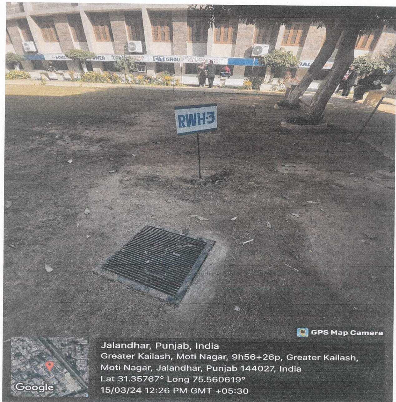
Rain water harvesting Pit
